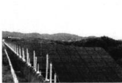
Array of panels on former maglev test track
